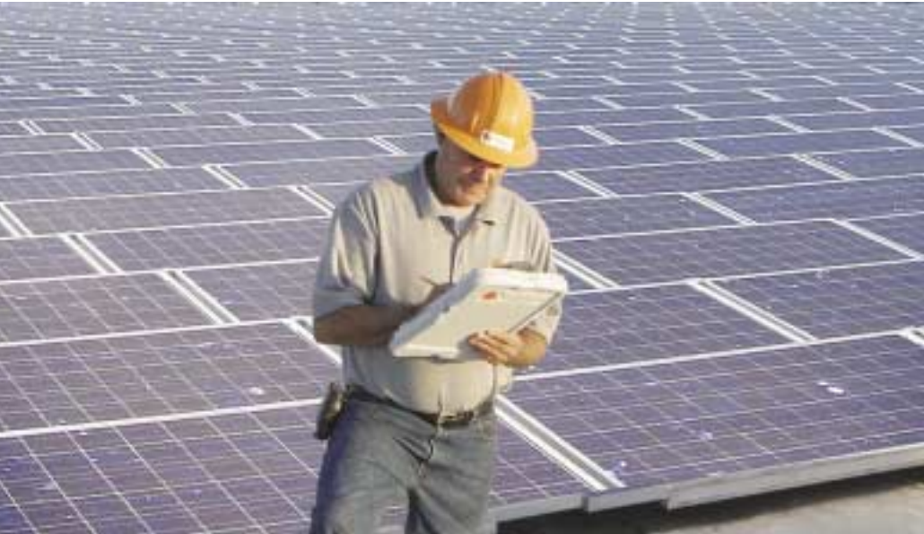
Early Morning Service, California Central Valley 1MW (AC)
